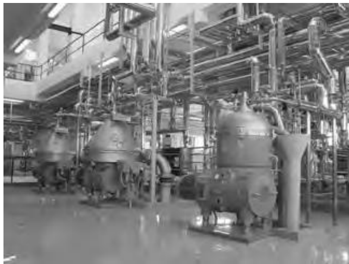
Figure 3.1: A piping network in an industrial facility.
